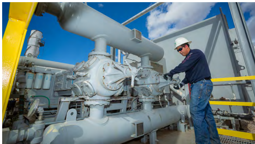
← Lucid’s Roadrunner cryogenic gas processing plant in Eddy County located near Loving, New Mexico
