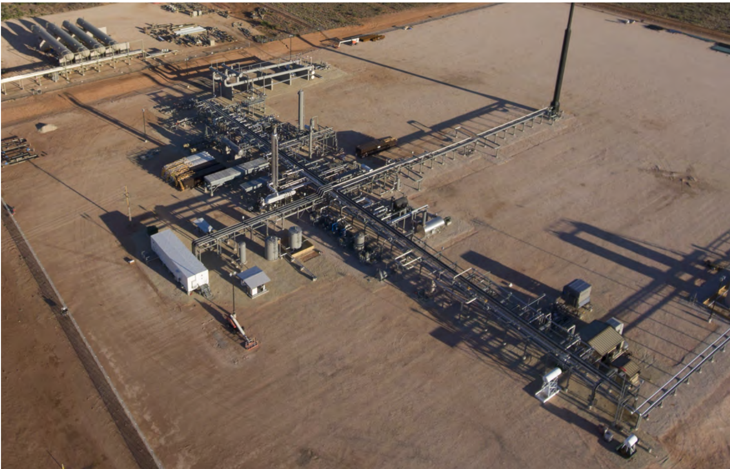
↓ Lucid's off-spec gas treating facility at Red Hills removes hydrogen sulfide from the gas stream and sequesters it by injection in a disposal well
