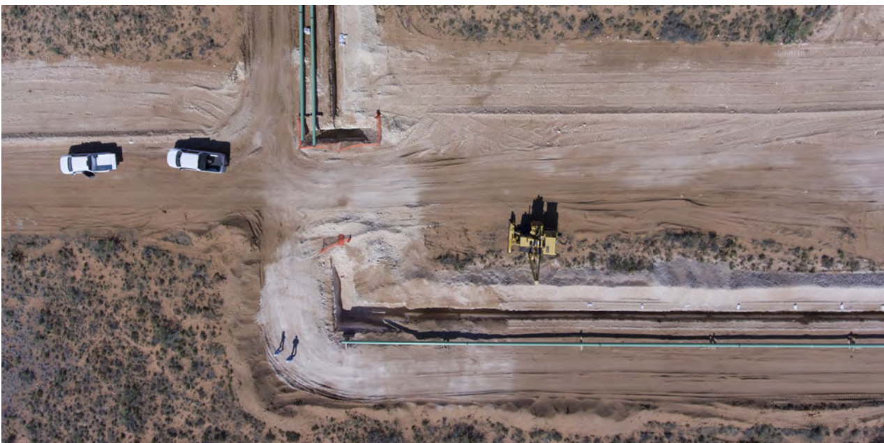
↓ Lucid project management teams lowering in a new pipeline with contractors as the gathering system expands
