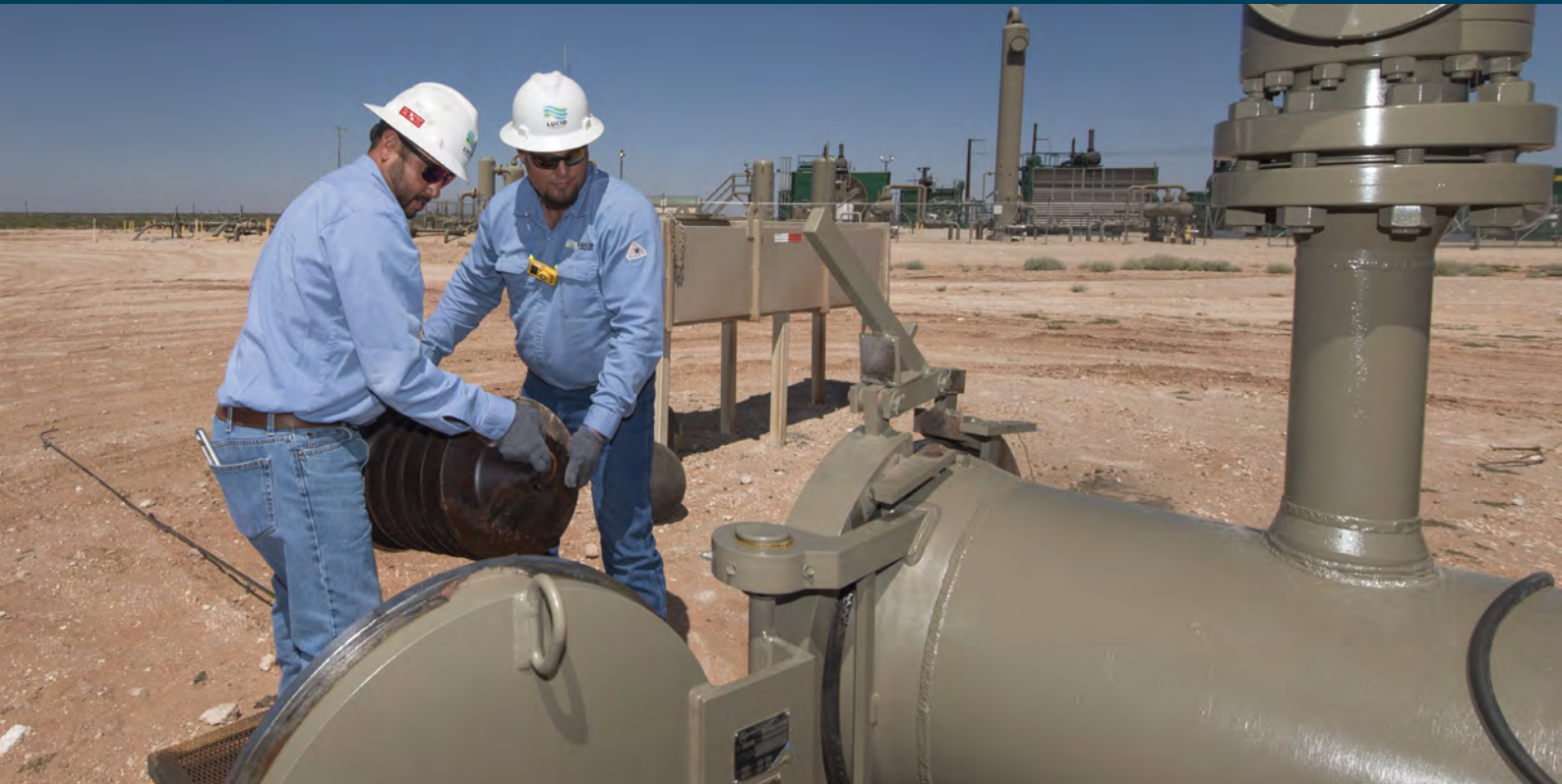
↓ Pipeline operating team members load a pipeline cleaning pig at the Frac Cat Compressor Station in Lea County New Mexico.
